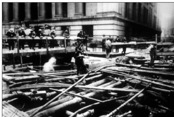
FIGURE 1 Underground infrastructure at Wall Street and Williams Street in New York City, 1917. Source: Consolidated Edison Company of New York, Inc.
