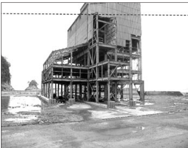
FIGURE 4 The La Farge Cement Plant was a well designed steel-framed structure anchored to rock. The metal siding was stripped from the buildings up to the wave-flow height of ~35 meters.
