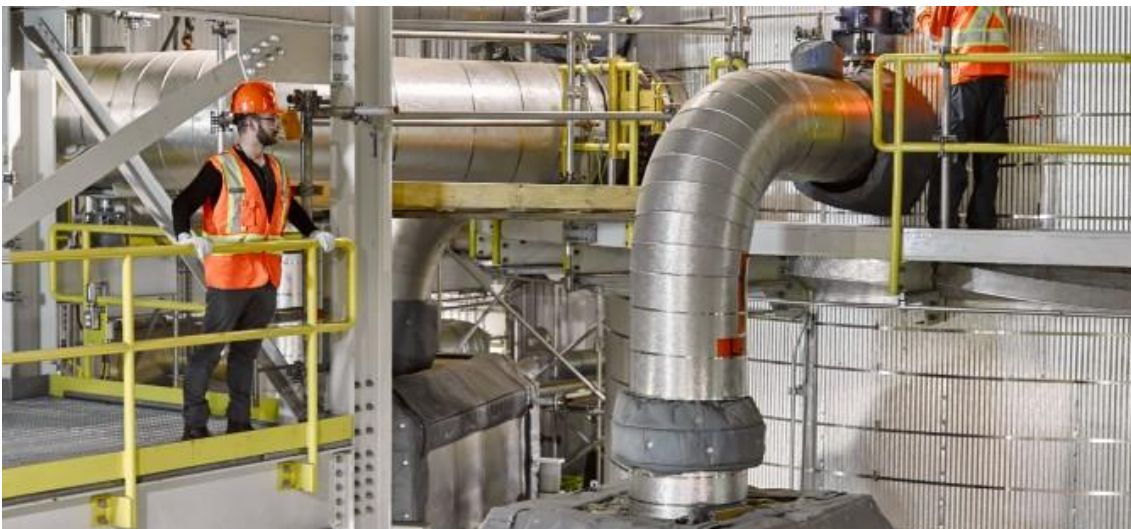
Figure 1 A carbon capture facility in Saskatchewan, Canada. Photo: SaskPower via a CC-BY-NC-SA 2.0 license
